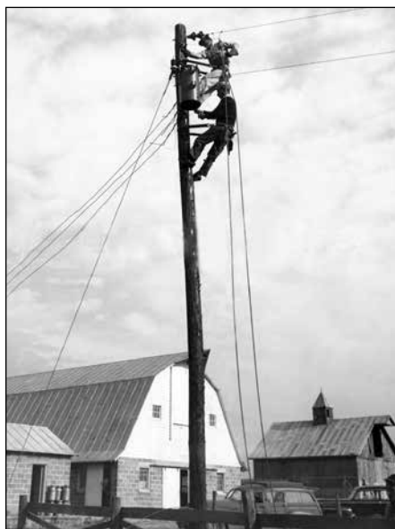
Cooperative linemen installing a transformer to serve a farmer at the end of a rural line extension.
