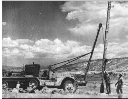
Showing a Garkane Rural Electric Cooperative line crew setting a pole with a home-made derrick in Southern Utah.
